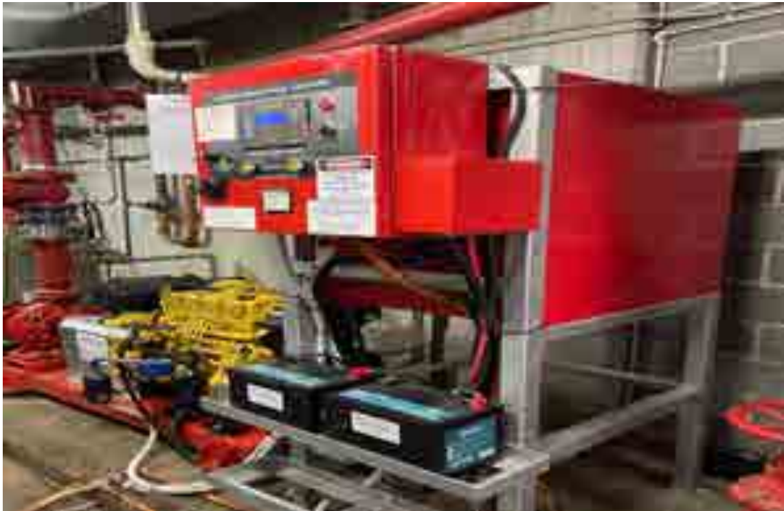
Photograph 2 Above-ground diesel tank within sprinkler / pump room
